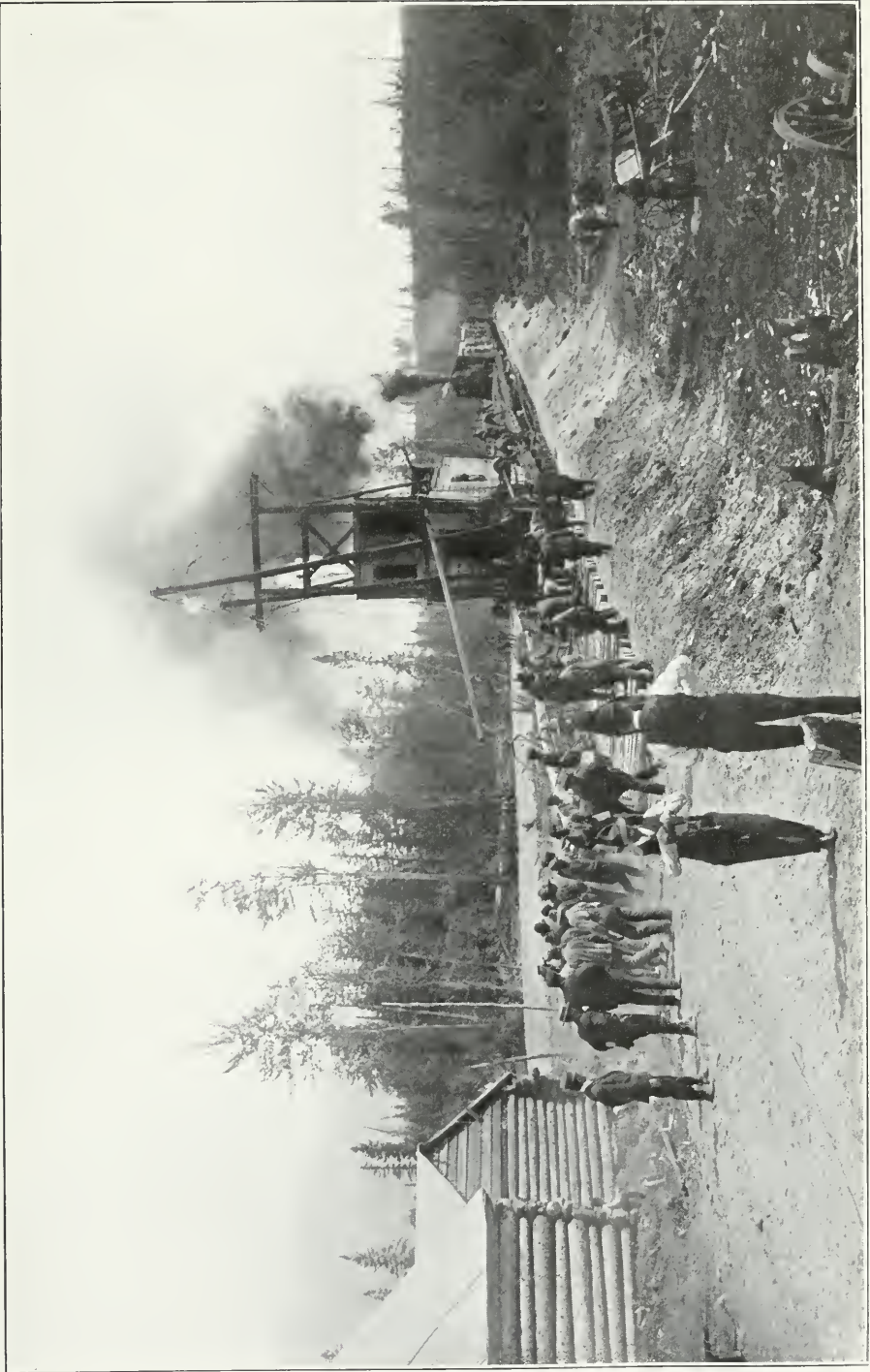
Grand Trunk Pacific Railway. Track laying machine coming into Tête Jaune Cache, B.C.
