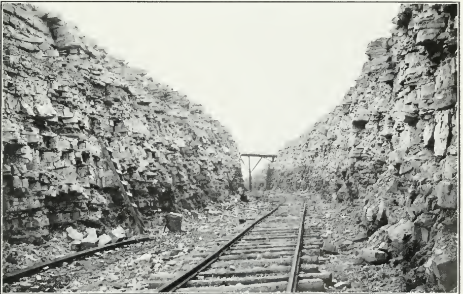
New Welland Ship Canal. Rock cutting for diversion of Grand Trunk Railway, Thorold.
